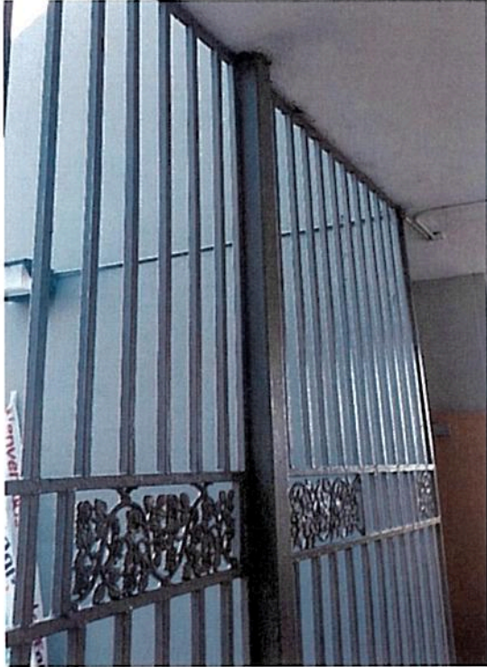
Photo #5 Corrosion of steel column in school.
